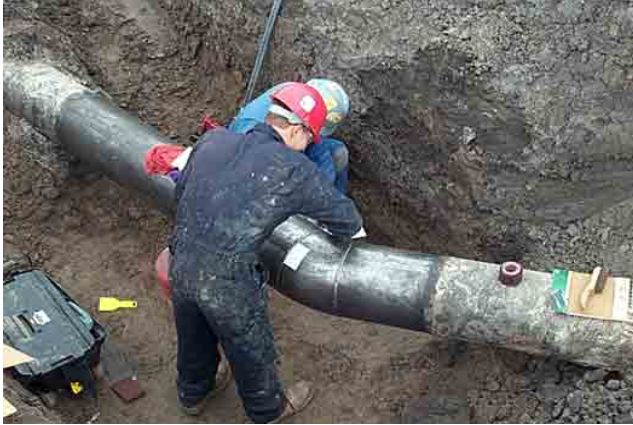
Each PermaWrap sleeve is cut, mitered to fit, and numbered at WrapMaster's facility. Prior to application, the individual PermaWrap sleeves are dry fitted and taped into position and checked for proper fit.
