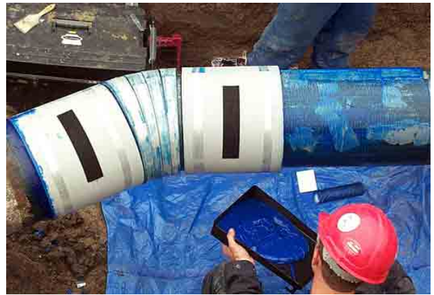
In the photo above, a sleeve is applied to both ends of the bend repair area, butted next to the girth weld. The void in the girth weld area will be filled using WrapMaster's PermaPutty high compressive filler material. Two PermaWrap sleeve will be applied over the girth weld areas to be reinforced.
