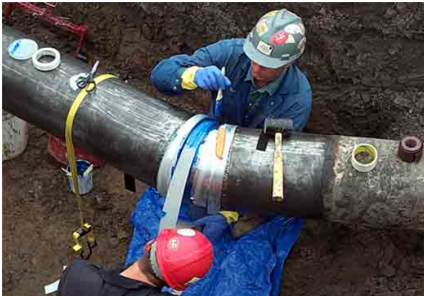
The excess PermaGrip adhesive and PermaPutty are removed from both edges of the installed sleeve. Using the same procedure, the remaining numbered sleeves are then applied.
