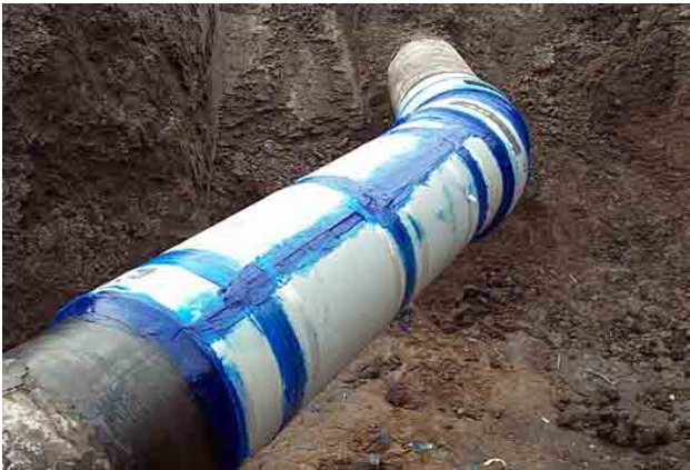
In the photo above, several PermaWrap sleeves were butted end-to-end to reinforce an area of general corrosion.
