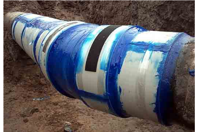
The photo above shows the completed bend repair area. As mentioned above, notice the P12-6 (12x6) PermaWrap sleeves installed over the girth weld for reinforcement.
